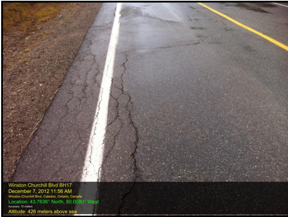
Figure 3 Winston Churchill Blvd. - Pavement Edge Break/ Severe Cracking
