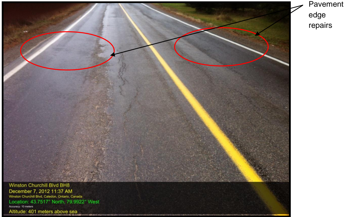
Figure 1 Winston Churchill Blvd. - General Pavement Overview, noting extensive edge repairs
