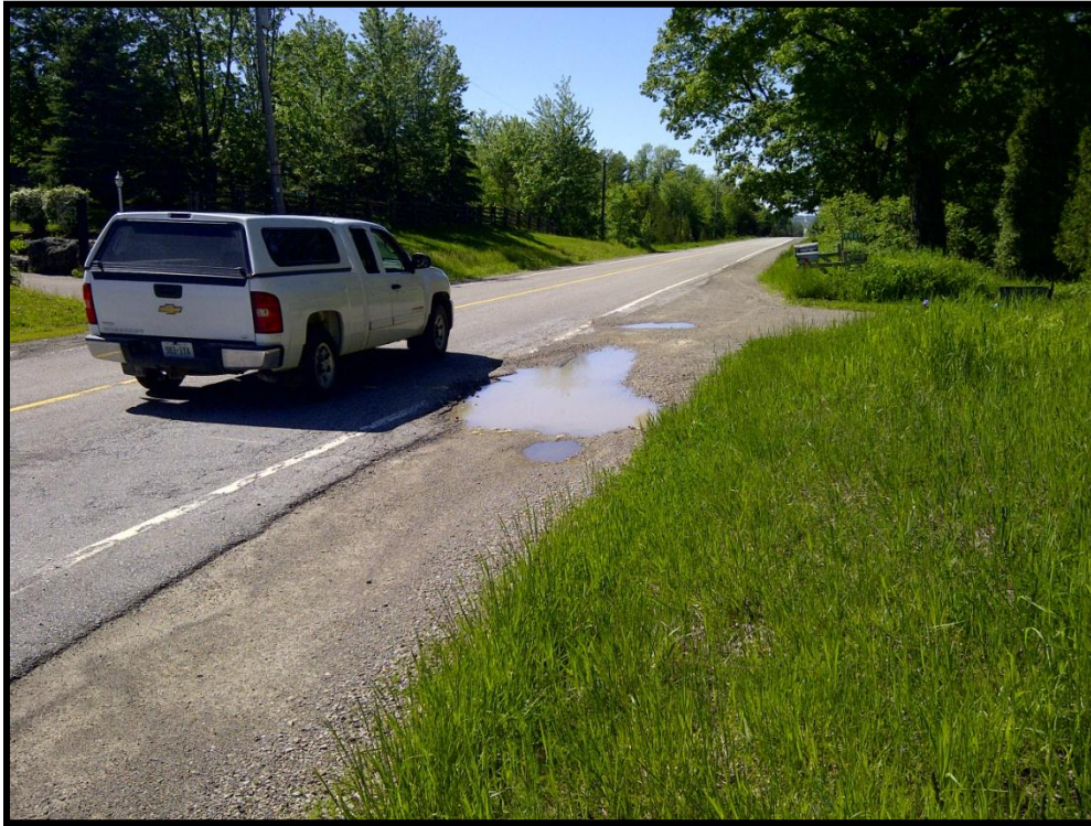
Figure 6 Winston Churchill Blvd. - Ponding in Shoulder - Faulty Grading near Pavement Edge
