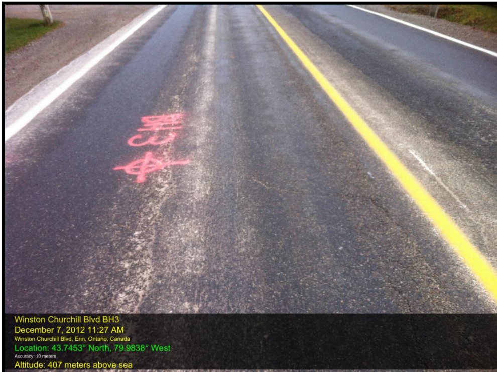
Figure 4 Winston Churchill Blvd. - Surface Distortion (Wheel Path Rutting), and Flushing
