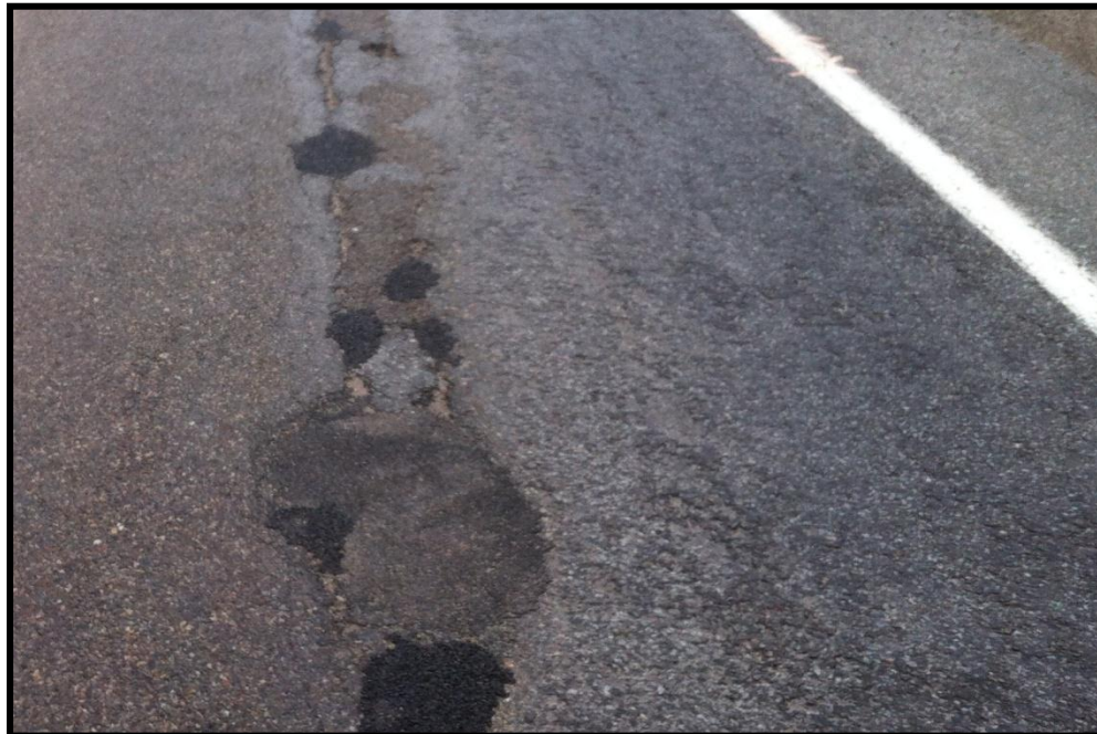
Figure 2 Winston Churchill Blvd. - Close up on Pavement Surface Condition: Failing Patch Work, Severe Ravelling
