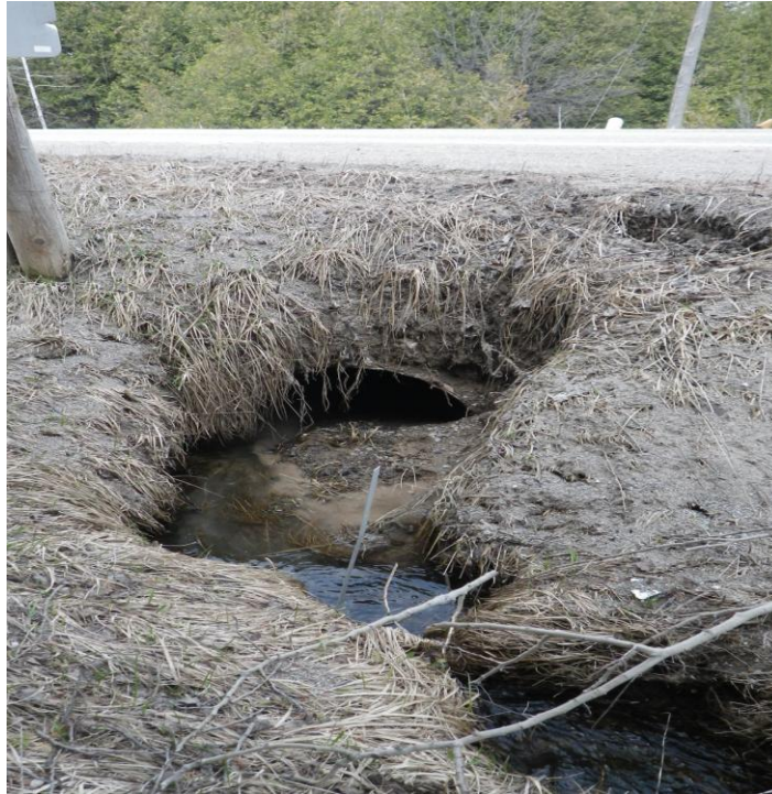
Photo 15: View looking upstream towards culvert inlet which is being compromised by the failing bank.
