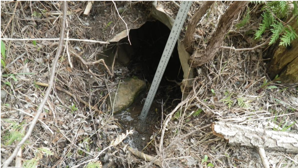
Photo 13: View looking downstream towards culvert inlet. Culvert appears to be collapsing.
