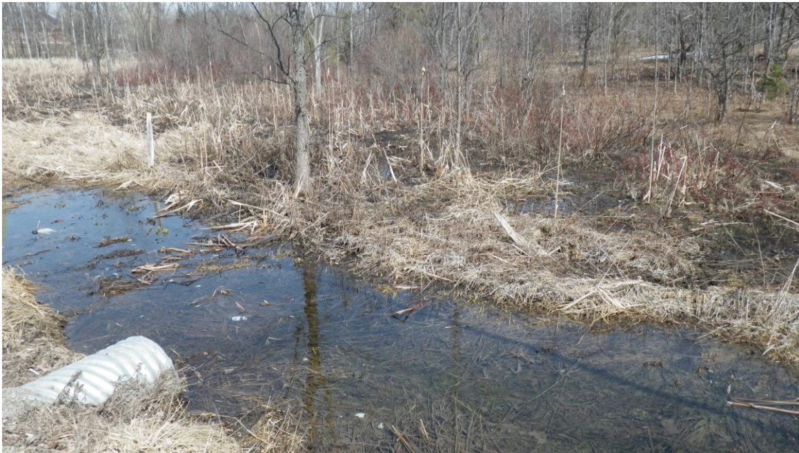
Photo 3: View looking downstream from culvert inlet where channel is undefined.
