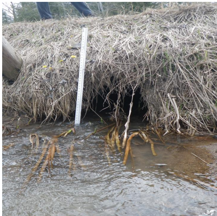
Photo 16: View looking upstream towards culvert outlet which is being compromised due to slumping bank.
